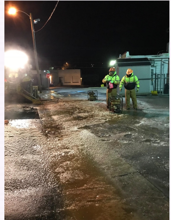
Main Break – Air Temperature 10°, Wind Chill below 0°
