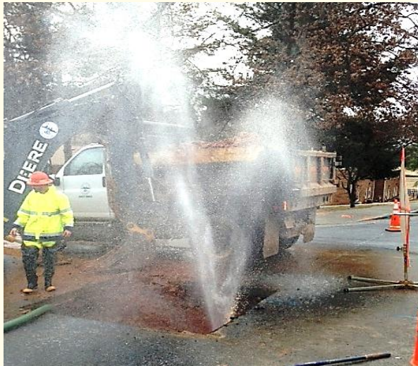
Water line Breaks
