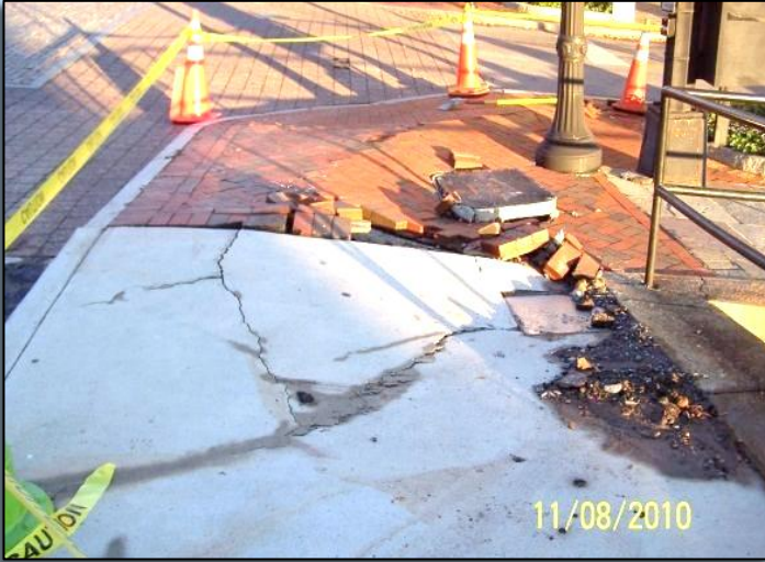
Water main break – damage to concrete and brick sidewalks.
