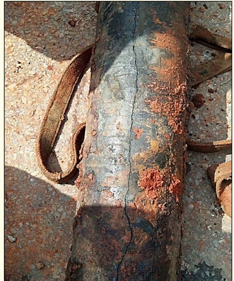
5 th Street – 8" Water Main
