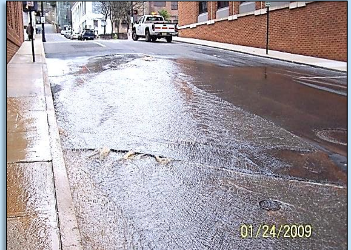
Water main break – damage to pavement.
