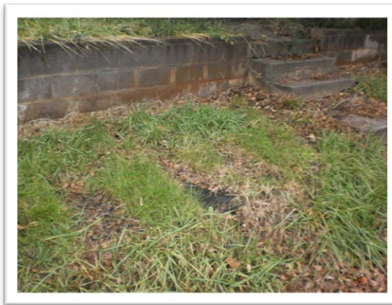
Sidewalk covered up over time
