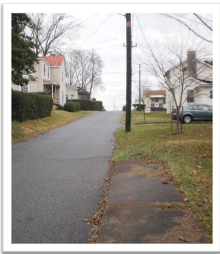
Possible to add missing sidewalk segment
