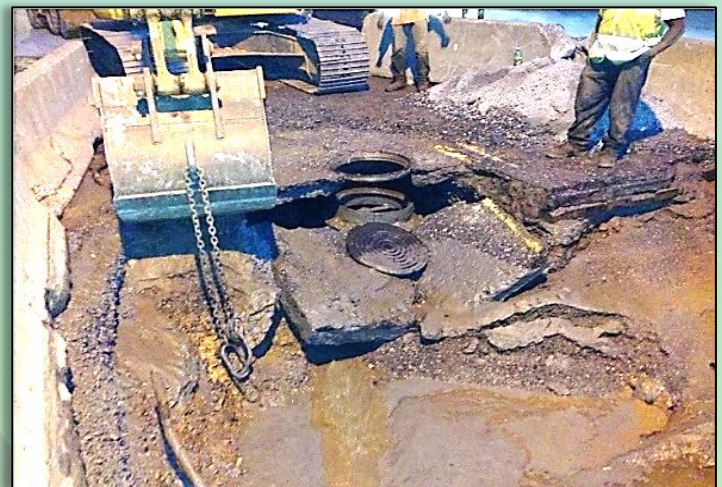
Water main break – damage to pavement and sewer manhole (risk of cross contamination from sewer)
