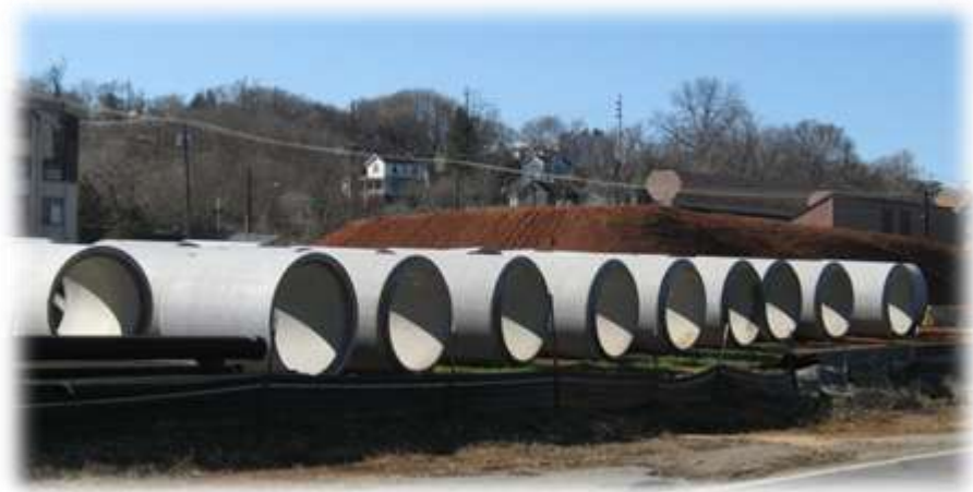
Pipe for James River Interceptor Division 3A
