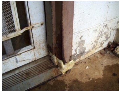
Graphic #17 – Rusting Door Frame
