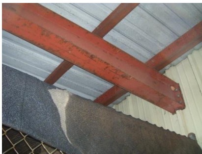
Graphic #6 – Rusting Structural Steel
