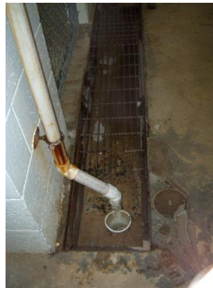
Graphic #25 – Steel Grate Over Trench Drain
