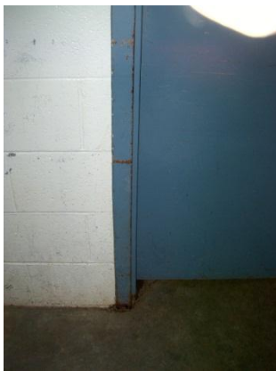
Graphic #18 – Rusting Door & Door Frame
