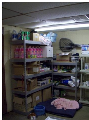
Graphic #15 – Sagging Acoustical Ceiling
