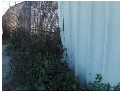
Graphic #5 – Damaged Metal Siding
