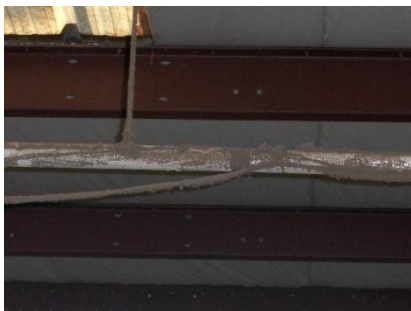
Graphic #26 – Dirt On Water Pipe
