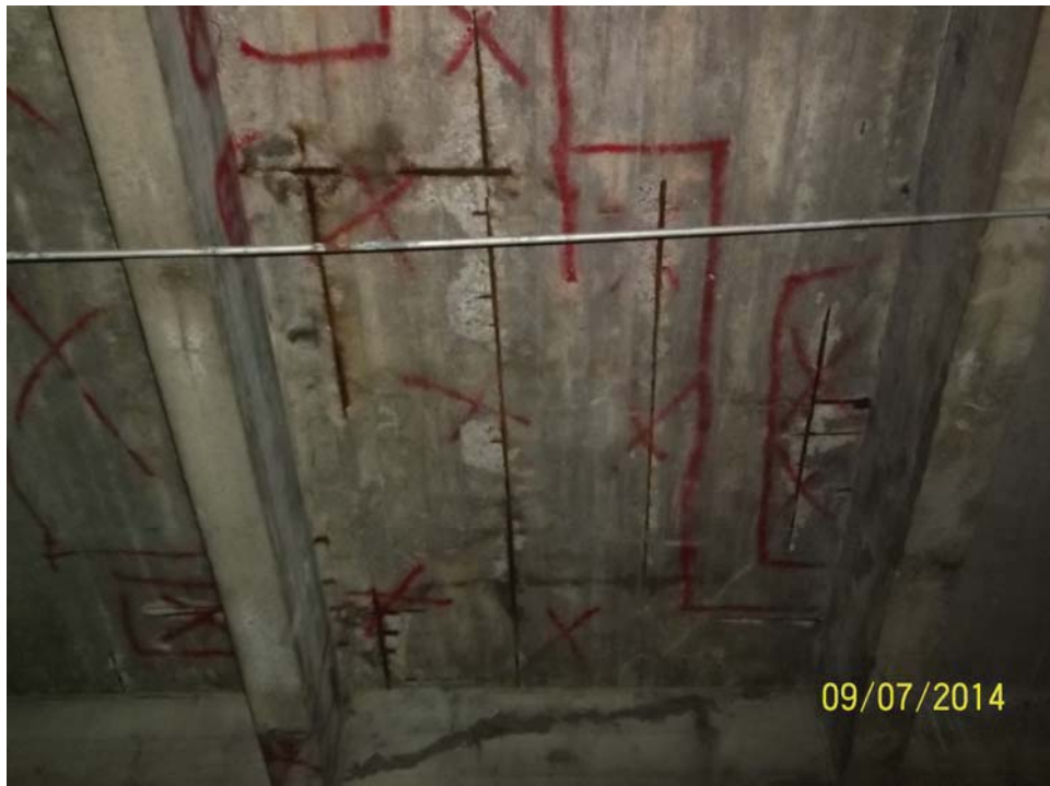
(14) Bay A1 panel 6 – Spalled and delaminated concrete with exposed reinforcing steel
