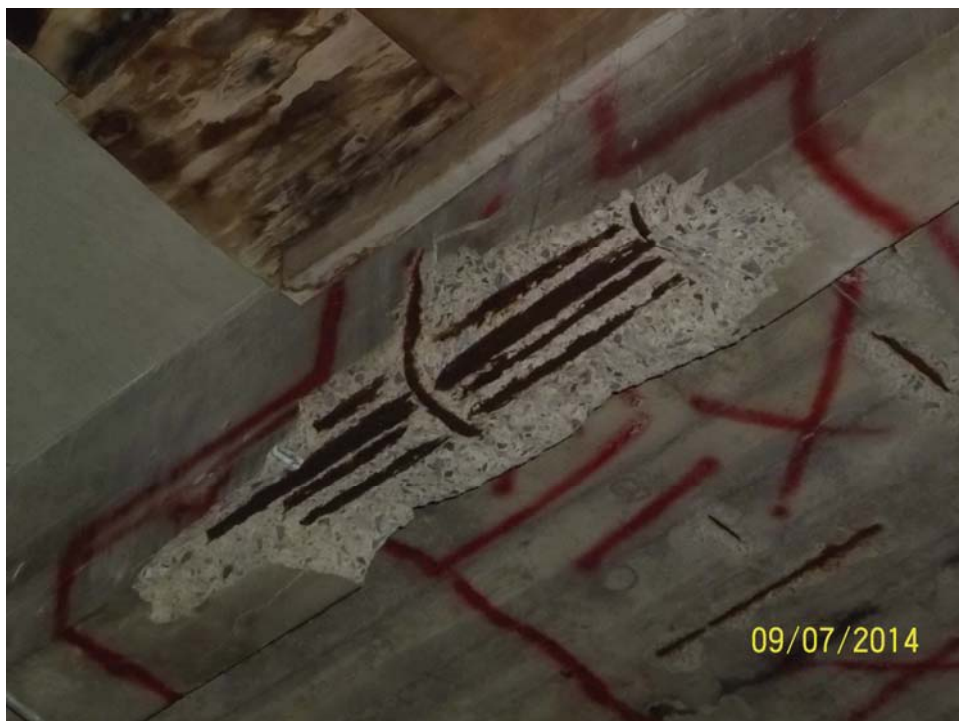
(15) Bay A1 panel 8 – Spalled and delaminated concrete with exposed reinforcing steel
