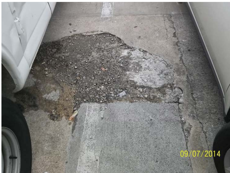
(3) Top of deck – Spalled and delaminated concrete
