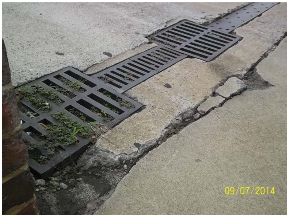
(6) Entrance – Clogged trench drain
