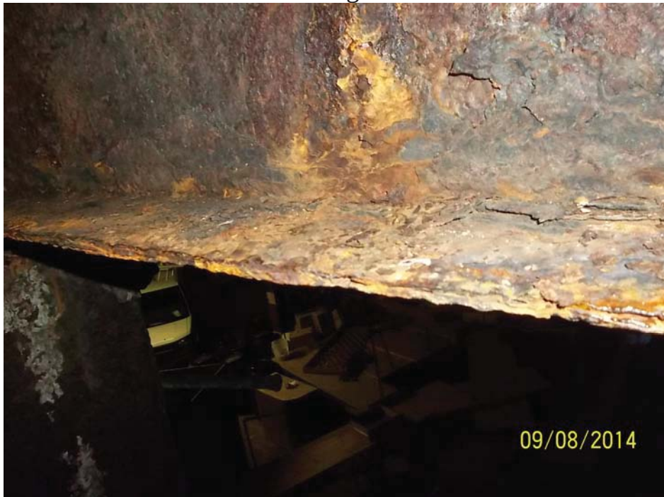
(30) Floorbeam 11A – connected to column CA has \frac{3}{16} " remaining in bottom flange for 4' and web has 75% section loss full height between stringer 1 and stringer 2
