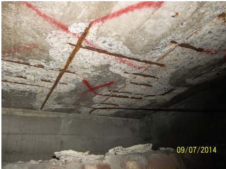
(24) Bay C, panel 2 – Spalled and delaminated concrete with exposed reinforcing steel
