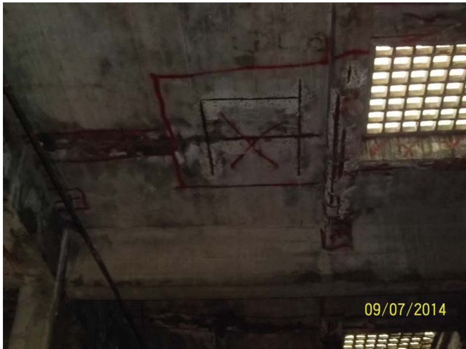
(26) Bay D, panel 6 – Spalled and delaminated concrete with exposed reinforcing steel
