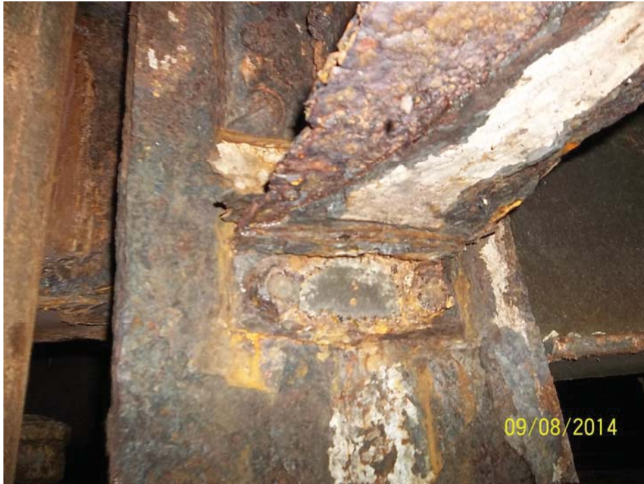
(31) Floorbeam 11A – clip angle under bottom flange has 90% section loss in top leg
