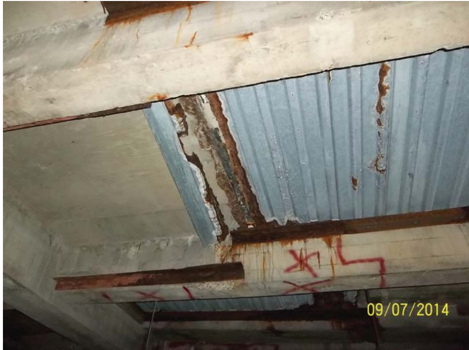
(21) Bay B panel 1 – Metal decking and delaminated beam
