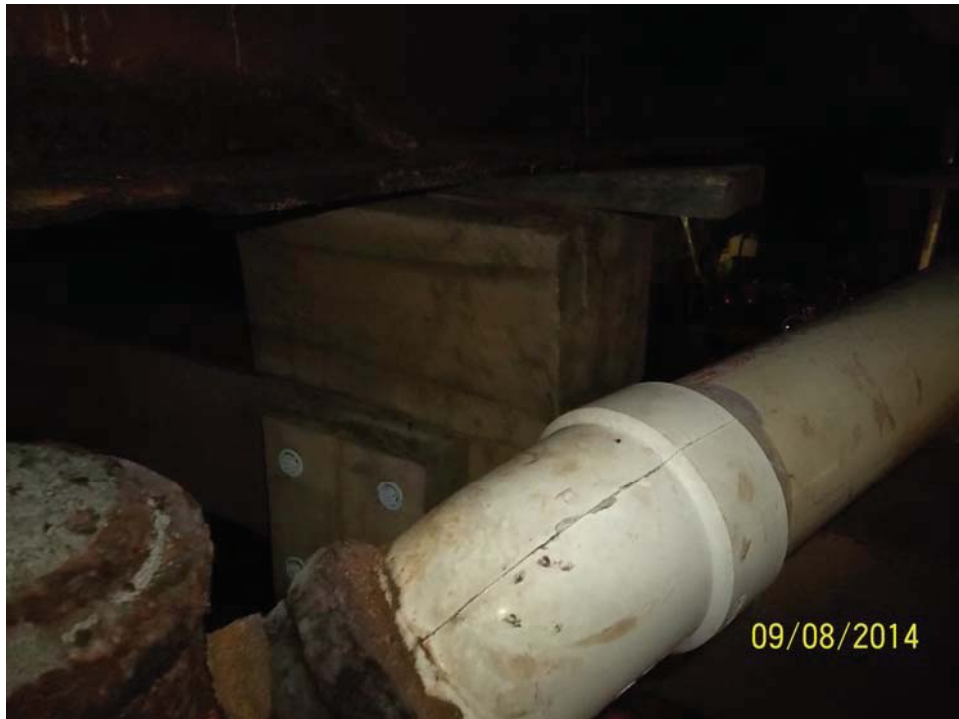
(19) Temporary seat block under stringer 2 – block is split
