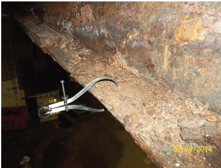
(34) Floor beam 11C – Has 1/8" section loss on bottom flange, 10' out from column CB, panel 10
