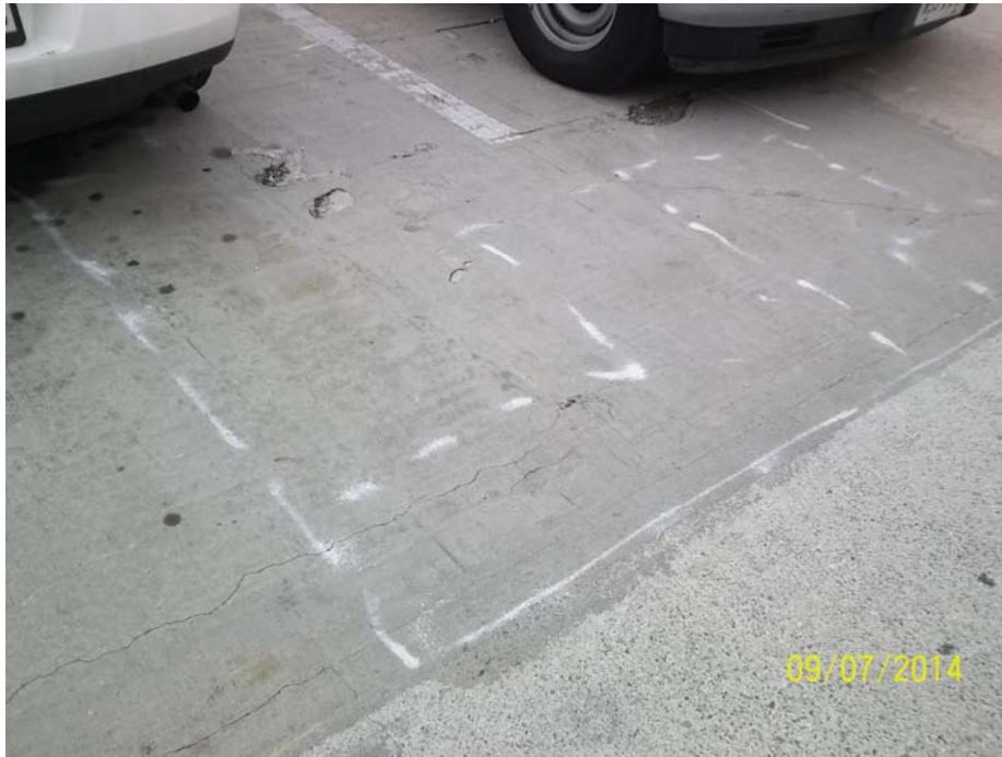
(1) Top of deck – Spalled and delaminated concrete
