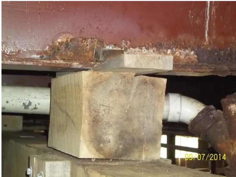
(18) Temporary seat block under stringer 2 – timber block not bearing on cap
