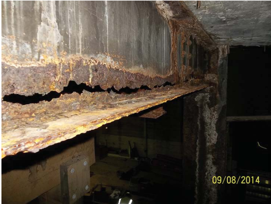
(29) Floorbeam 11B – web between column CB &CA has a corrosion hole 4" high full length along bottom
