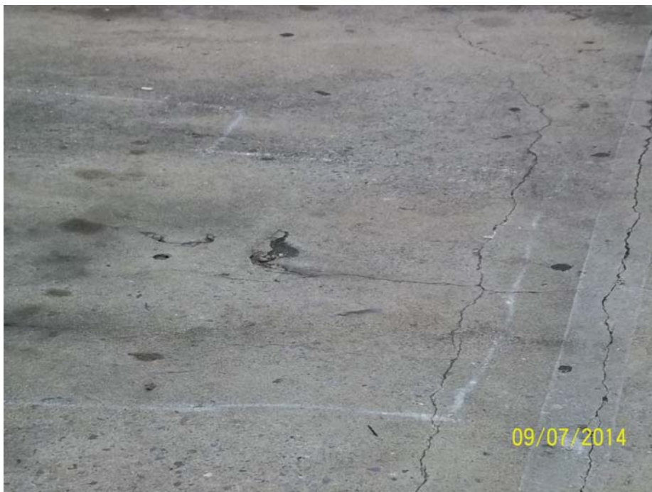
(2) Top of deck – Spalled and delaminated concrete
