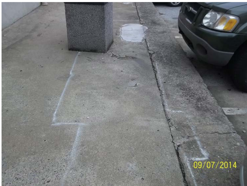
(4) Top of sidewalk – Spalled and delaminated concrete
