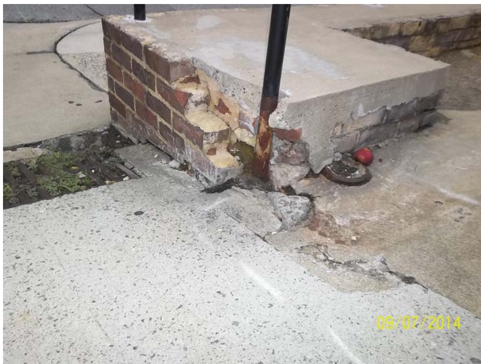
(5) Entrance – Spalled concrete and broken handrail
