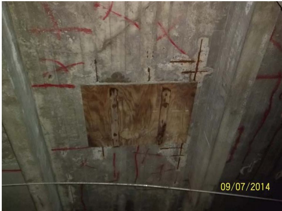
(13) Bay A1 panel 4 – Spalled and delaminated concrete with exposed reinforcing steel
