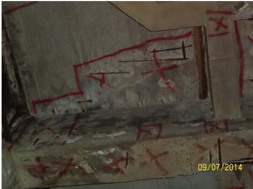
(25) Bay C panel 9 – Spalled and delaminated concrete with exposed reinforcing steel
