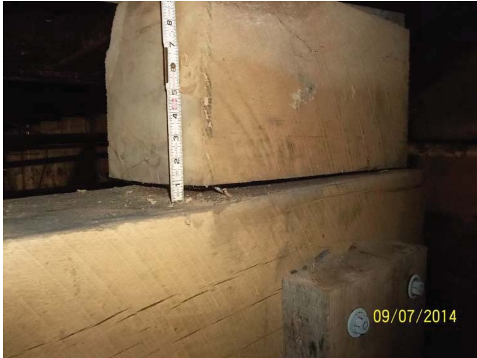
(17) Temporary seat block under stringer 1 – timber block not bearing on cap
