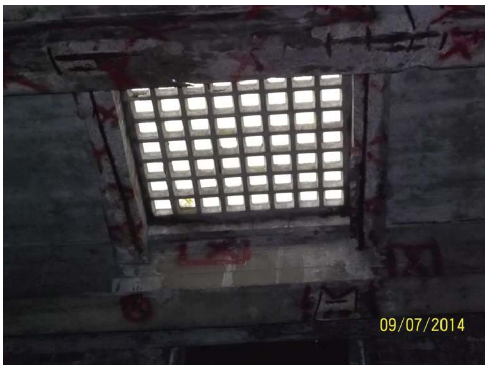
(28) Sky light – Spalled and delaminated concrete with exposed reinforcing steel
