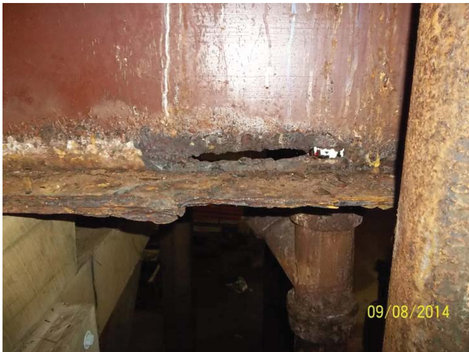
(32) Panel 10 stringer 2 – bolt flange has 50% section loss end 2' at column CA and web has 80% section loss in bottom 3" with 1" dia. Corrosion hole, 1' long for 2' at column CA
