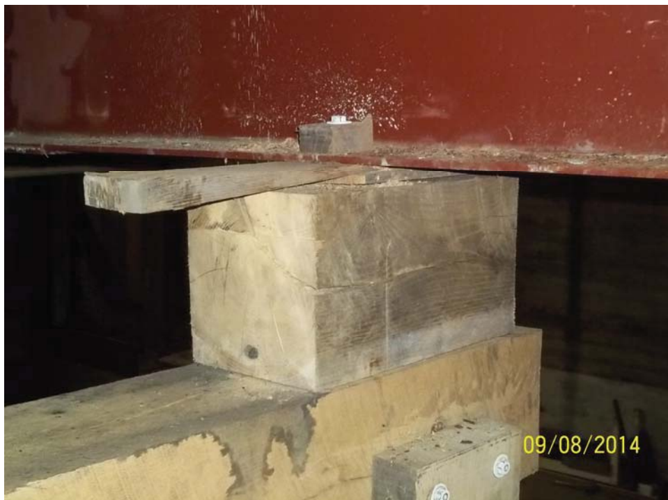
(20) Temporary seat block under stringer 3 – block is split
