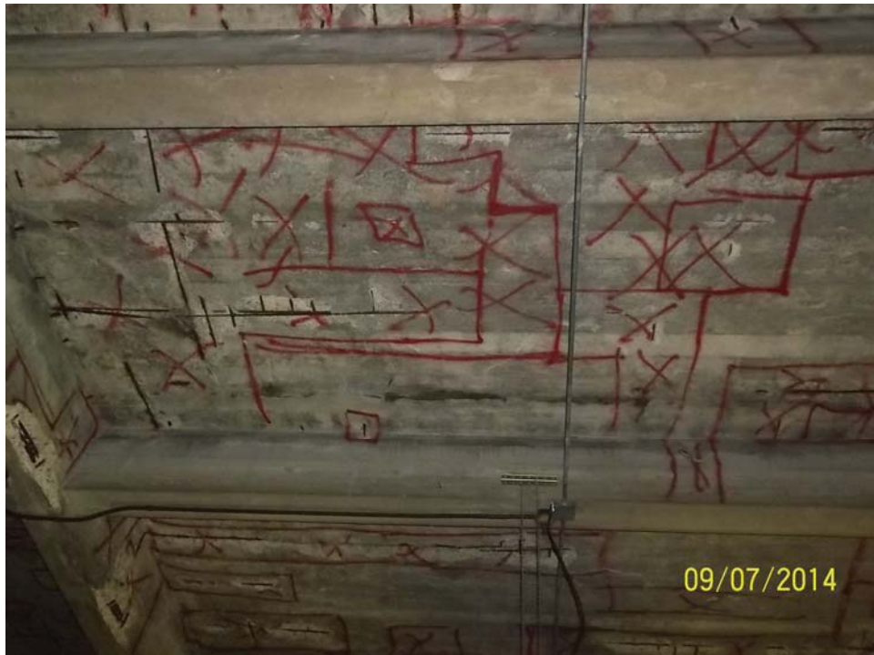
(23) Bay B, panel 8 - Spalled and delaminated concrete with exposed reinforcing steel
