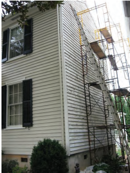
Original siding should be repaired and repainted as necessary (503 Washington Street).
