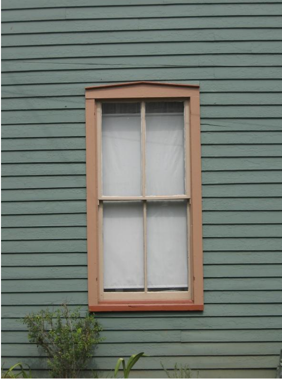
Window trim and moldings should not be removed or concealed (1225 Clay Street).
