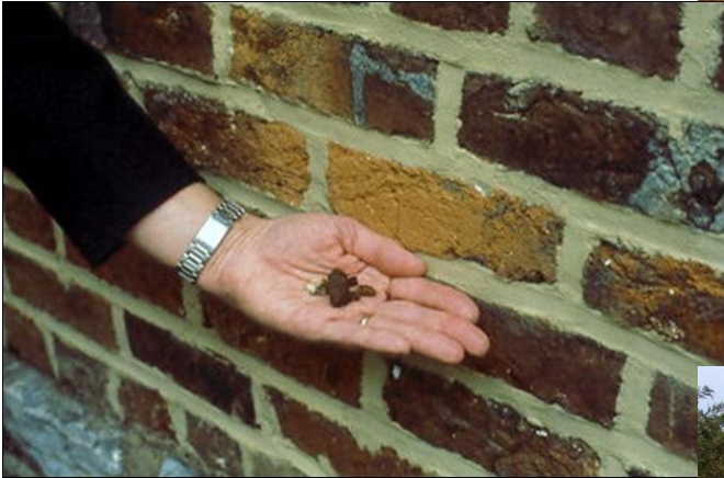
...leading to cracking and spalling.
