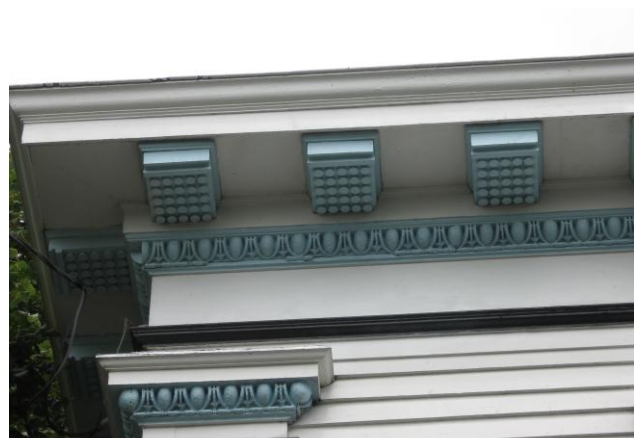
Eave decoration should be repaired or replicated using materials to match the original in texture, profile and appearance (405 Washington Street).
