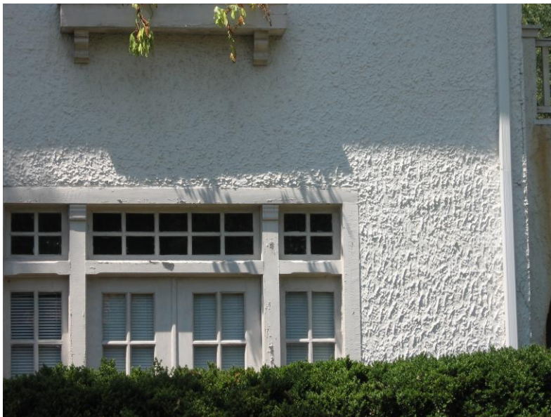
Exterior materials such as stucco should be repaired as needed and preserved (2312 Rivermont Avenue).
