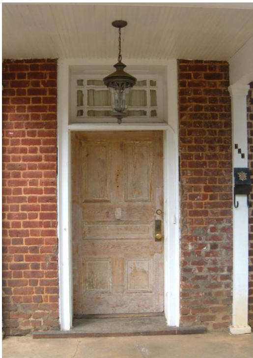
Original doors should be repaired and restored (223 Harrison Street).
