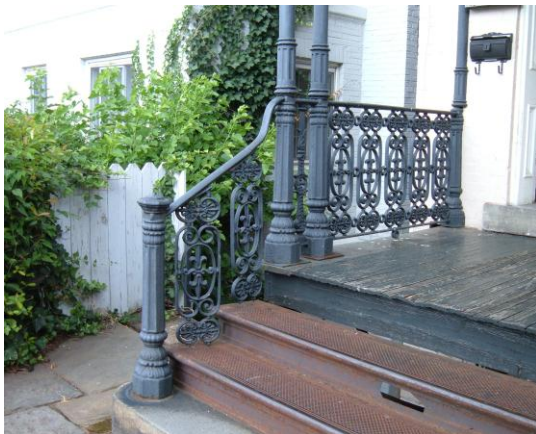
Cast iron railings should be preserved and maintained (708 Court Street).
