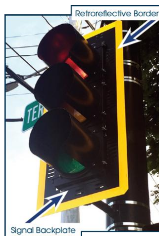
Figure 27: High-Visibility Signal Backplates. Source: FHWA
