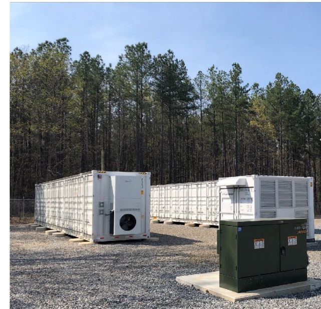
Rappahannock Electric Cooperative Project
