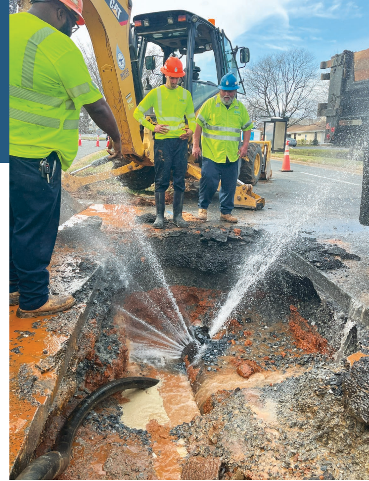
Water main break on Tate Springs Rd
